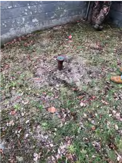
Photograph 3: UST fill pipe outside concrete block manufacturing building.
