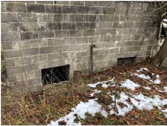
Photograph 37: Vent pipe and fill pipe for UST outside boiler room building.
