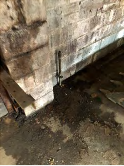
Photograph 19: Pipe below suspended AST.
