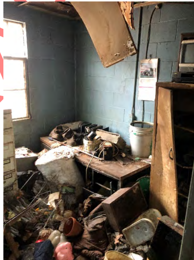
Photograph 84: Debris inside Dahlstrom office.
