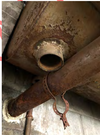
Photograph 18: Empty suspended AST in former dry-cleaning building.
