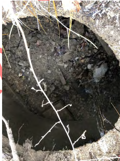
Photograph 72: Valve for public water supply.
