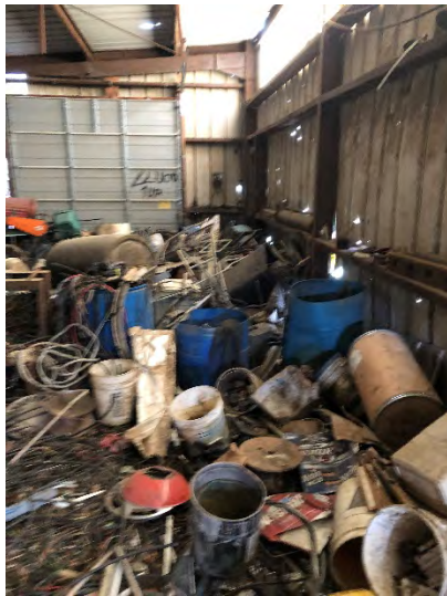
Photograph 87: Debris and scrap in Dahlstrom garage.
