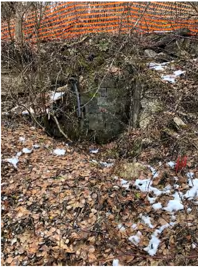
Photograph 73: Unknown pipe exiting bank on east side of Kraft property.
