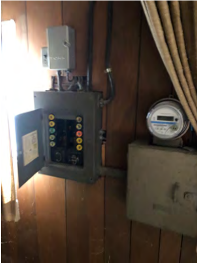
Photograph 23: Electrical in former dry-cleaning building.
