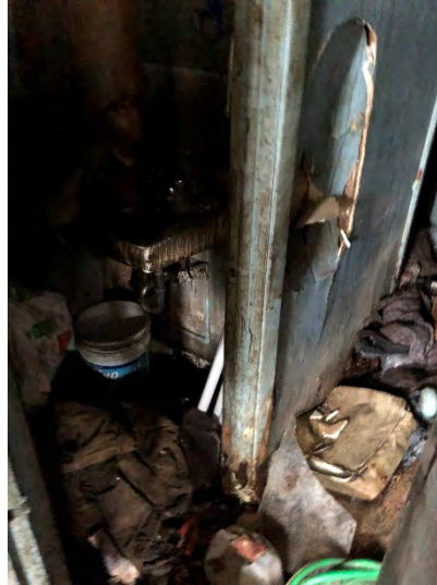
Photograph 82: Debris inside Dahlstrom office.
