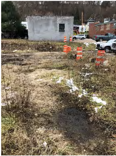
Photograph 105: Staining on Kraft property.
