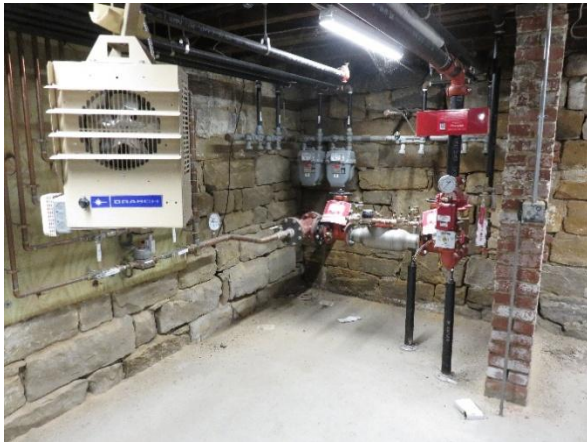
Fire Suppression Controls; in RFP, Need to extend to include 2 nd & 3 rd floors.
